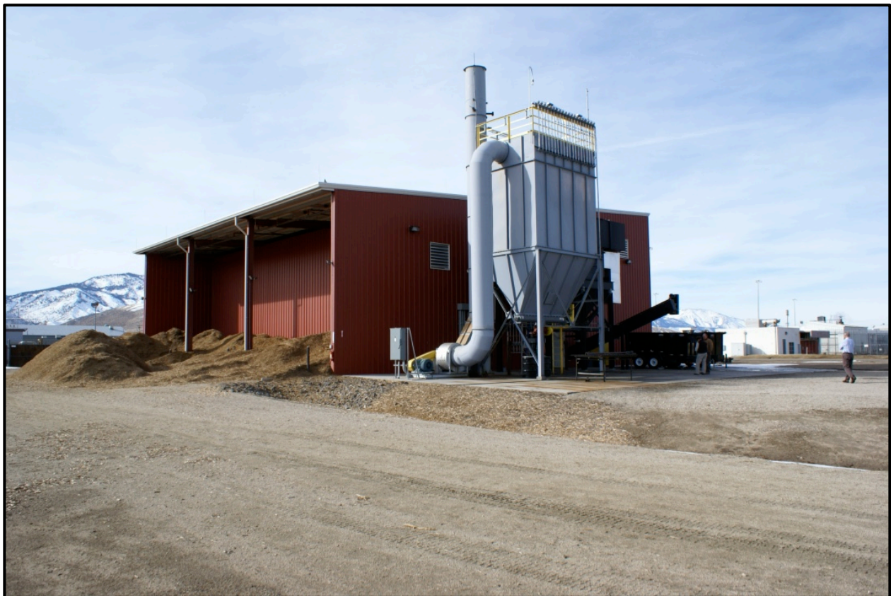
Small Direct Combustion Biomass Plant in Carson City, NV (currently offline)
