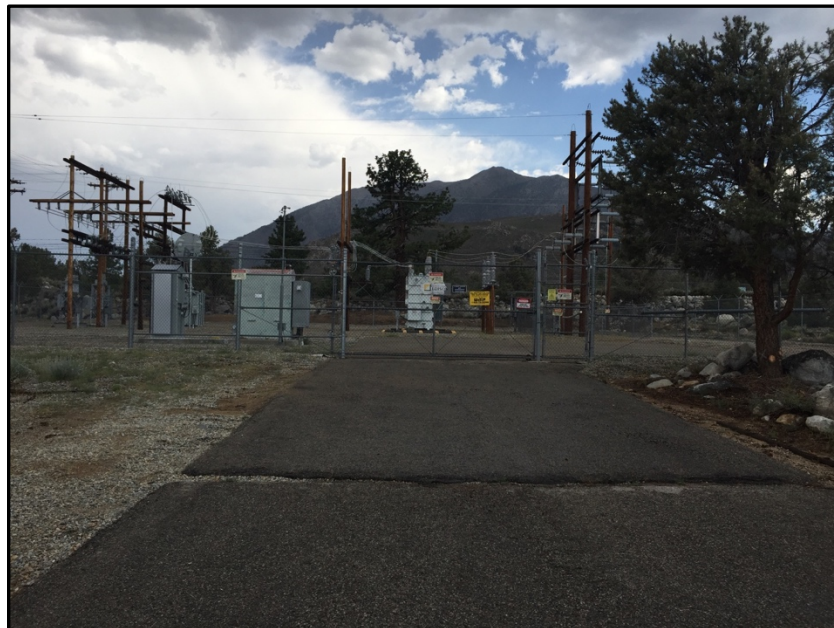
Figure 17. Tom's Place Substation
