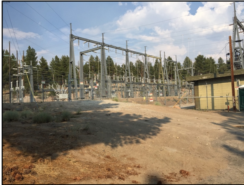
Figure 15. SCE Substation at Casa Diablo
